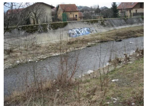
Figure 3. Concrete wall constructed in the years 1960 to reinforce the upstream face of the left rim embankment
