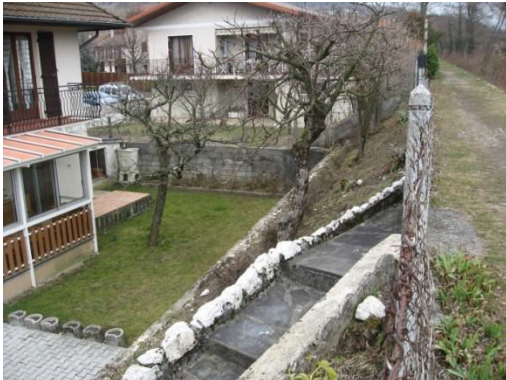
Figure 4. Retaining wall constructed without respecting the state of the art rules for that kind of structures
