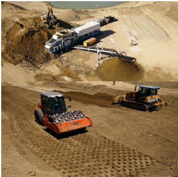
Figure 3. Mobile lime treatment plant (above) ; placement of treated soil and compaction by sheepfoot roller (below).
