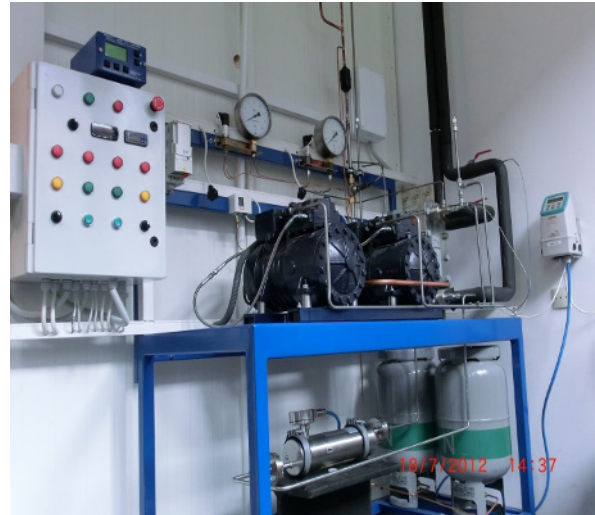
Figure 6. The LT refrigeration compression stage with mass flow meter below, and compressor control case.
