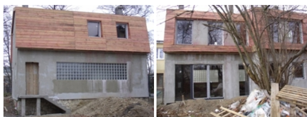
Figure 3. Improperly designed new building. a. south-western façade without glazing, b. northern façade – fully glazed, Kraków, Zarzecz street (photo by: W. Sobczyk)
