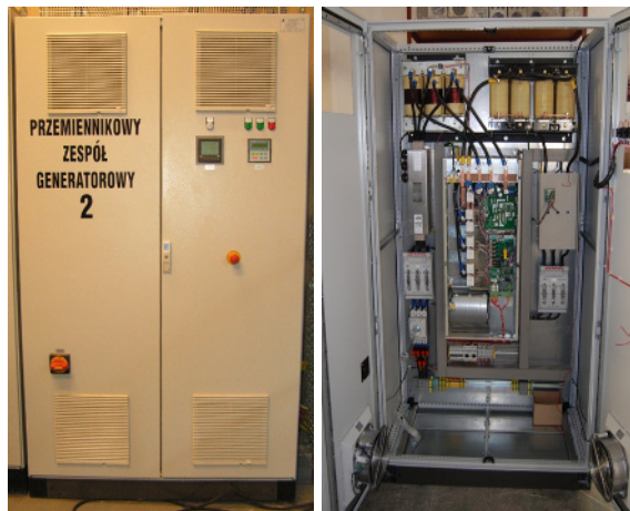
Figure 5. The view of the real power electronic converter of 90kW power.
