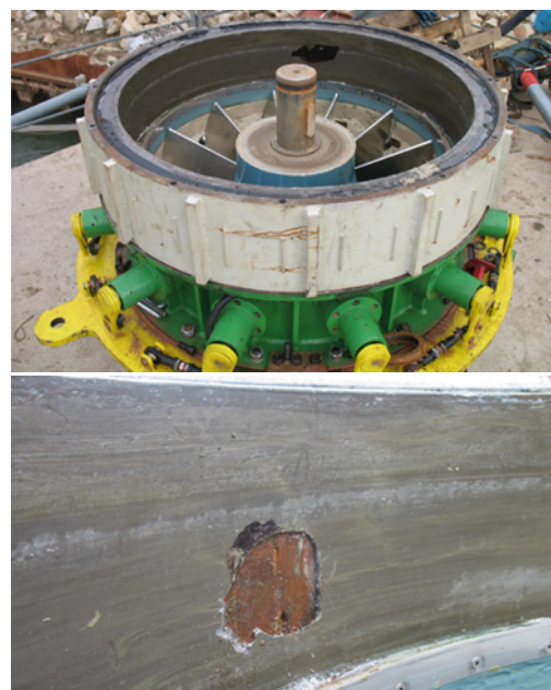
Figure 13. Insulation fault of the generator stator.
