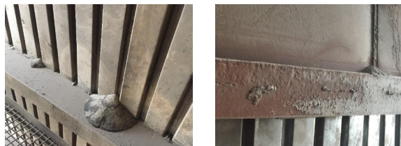
Figure 1. Damage of the isolation layer spotted on the analysed power boiler OP-140.
