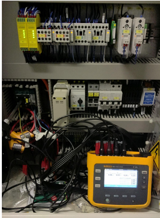
Fig. 3. Fluke logger connected to the Formiga P100
