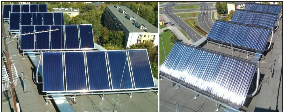
Fig. 1. Flat plate solar collectors connected in series of 5 units in one section (left side of the fig.), and evacuated tube solar collectors connected in series of 3 units in one section (right side of the fig.).
