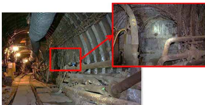
Fig. 2. Place of transverse leakage
