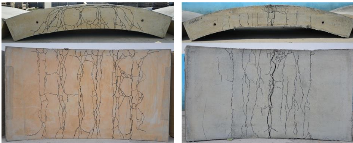
Figure 6 The crack pattern and failure morphology (Left: RC segment; Right: UHPFRC segment)
