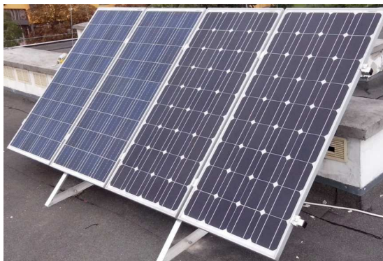
Fig. 1. Photovoltaic PV generator: left side polycrystalline PV modules - CL-130-12 model, and right side PV monocrystalline modules – AEMF 130 model
