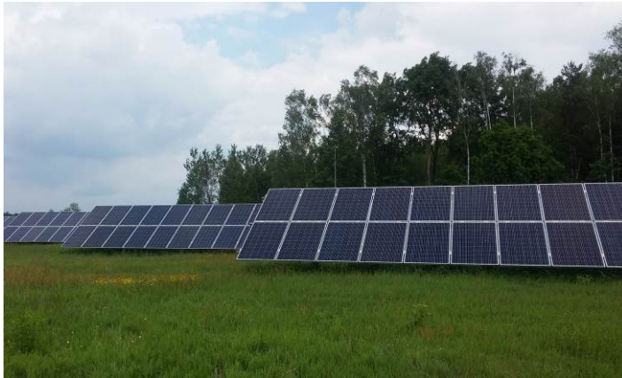
Fig. 1. Photovoltaic power plant of Zielawa Valley [the authors’ archive].
