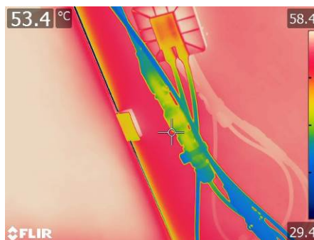
Fig. 11. Overheating occurred due to poor contact inside connector.
