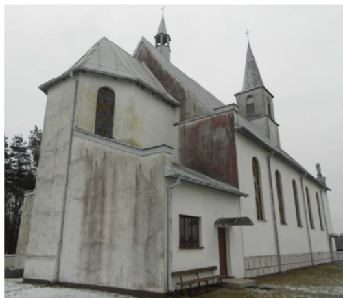
Fig. 7. Fungus on the outside wall. Source: own collection.
