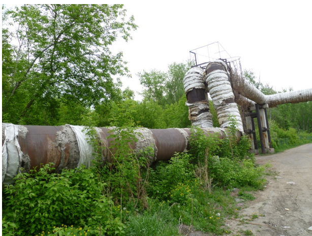
Fig. 4. Length with poor insulation.
