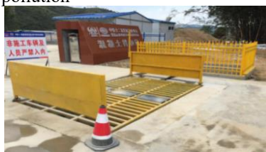
Figure 9. Automatic car washing device and wheel washing pool at the entrance and exit of mixing station.
