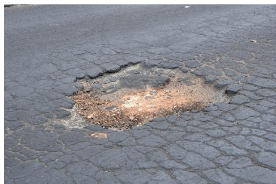
Fig 3. Fall of blocks from the pavement
