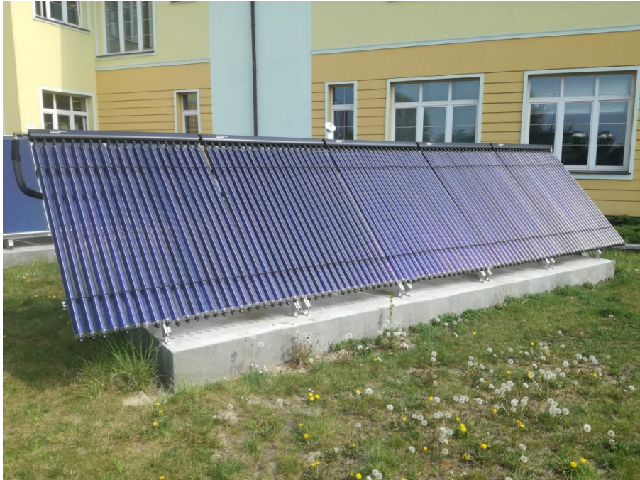
Fig. 1. Solar heating installation.
