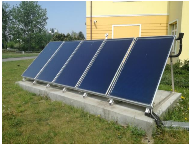
Fig. 2. Diagnosed solar water heating system.
