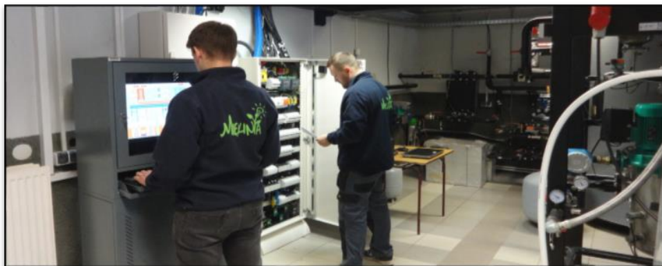
Fig. 4. Heat pump efficiency testing stand
