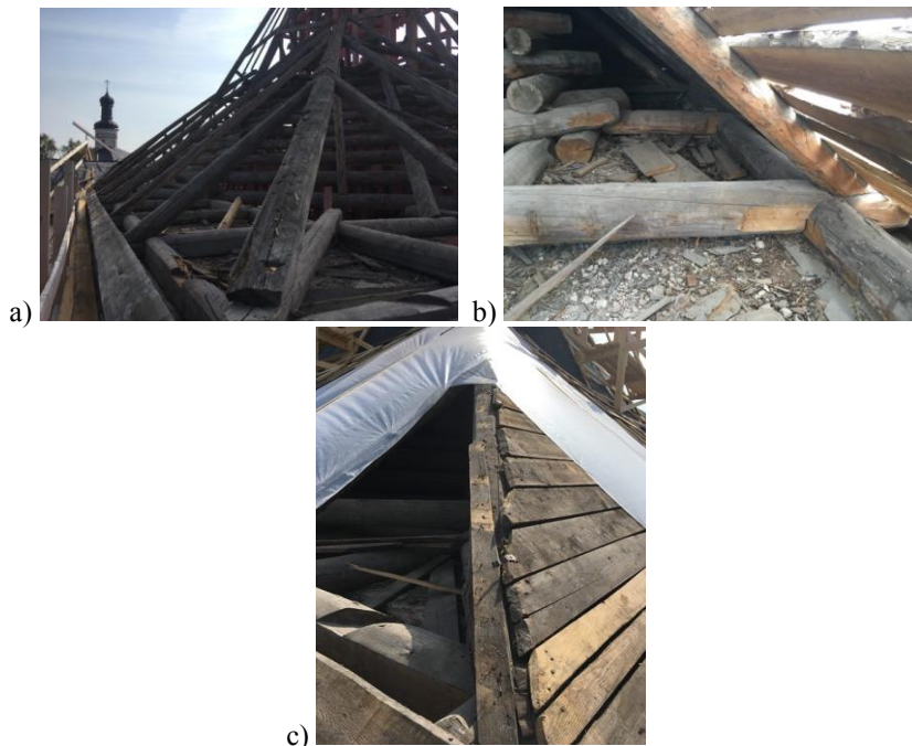
Fig. 7. Condition of the roof. The author of the photographs is Zhivotov D. A.: a) - the place where the cribbed structure is leaning on the walls; b) - existing and identified double wall plate; c) - condition of the crate.
