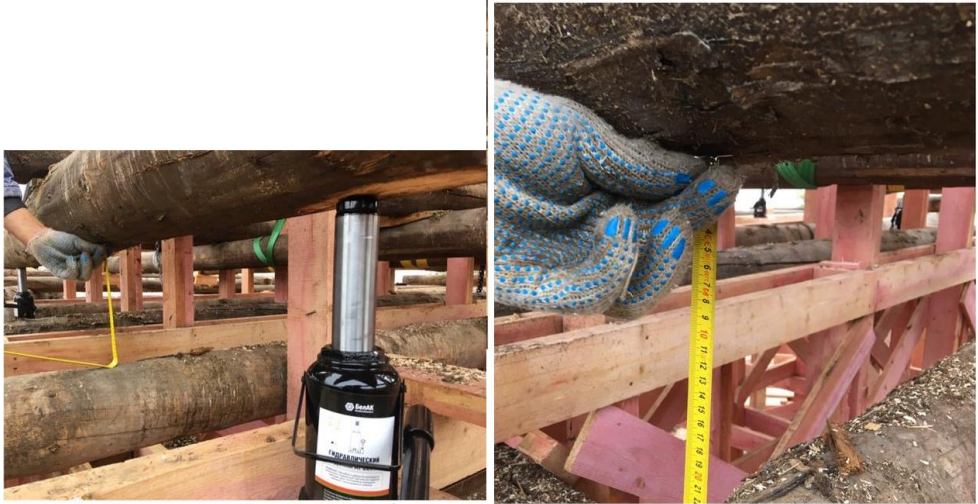
Fig. 12. Arrangement of jack for lifting the roof of the tower. The author of the photographs is Zhivotov D. A.
