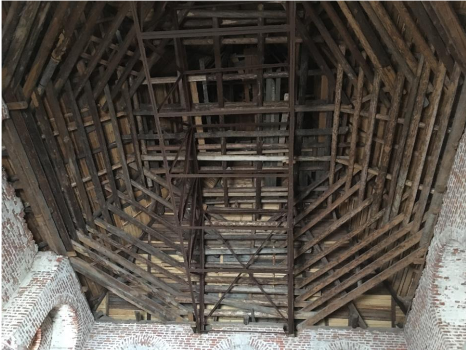
Fig. 4. A cribbed structure of hipped roof and a supporting metal truss installed in the 1970s. The author of the photos Galaktionova O. S.
