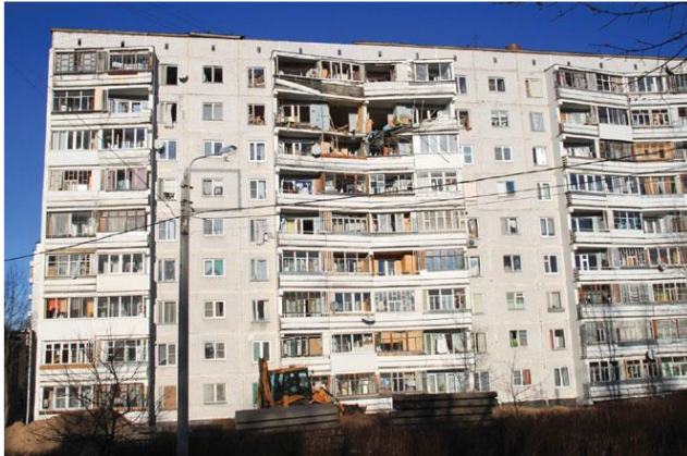
Fig. 2. General view of the affected building from the side opposite the entrances.
