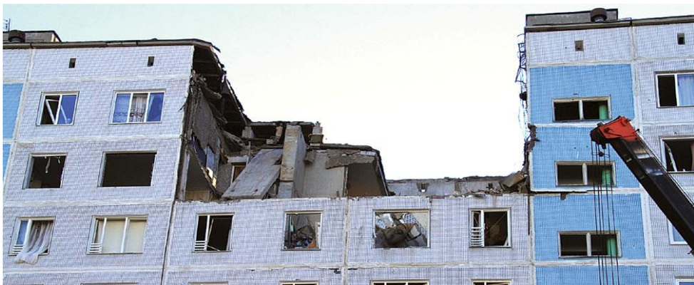
Fig. 1. Destroyed part of the building from the entrances.
