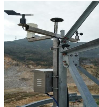
Fig. 3. Physical picture of iron tower and receiver near Nanjing railway station
