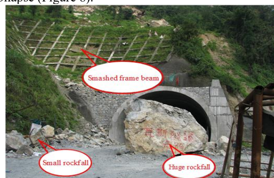
Figure 8. Rockfall and broken frame beam
