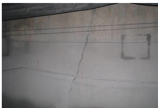
(a) Transverse and oblique cracking of the lining
