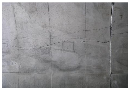
(b) Longitudinal cracking of the lining
