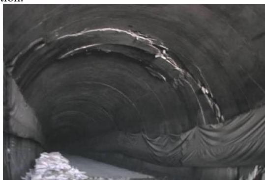
Figure 14. Circumferential crack in the bedrock-overburden interface
