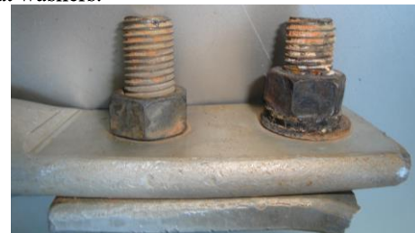
Fig. 10. Morphology of the failed clamp bolt.
