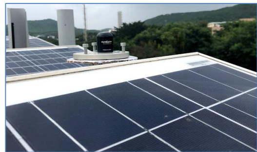
Fig. 4. Apogee SP110SS Pyranometer on terrace
