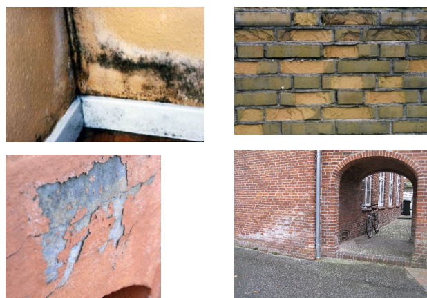
Fig. 3. Examples of visually apparent moisture induced damage of internal or external façades. From top left and clockwise: Mould growth at indoor surface, spalling due to frost, salt efflorescence, scaling of paint.
