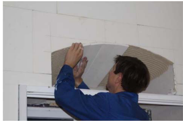
Fig. 9. Applying insulation on a rounded area at the window head reveal / Benediktbeuern.
