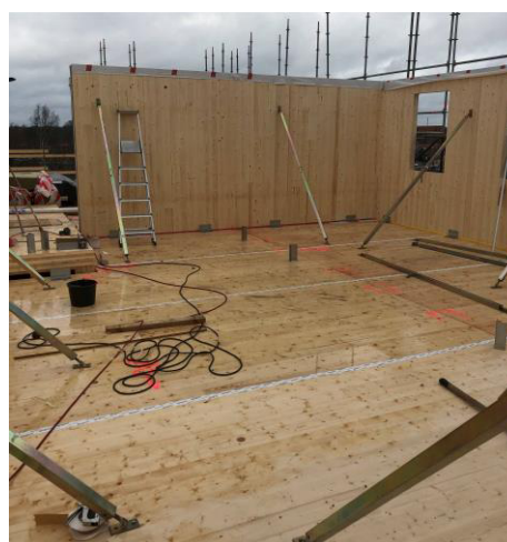
Fig. 3. Ongoing assembly with water standing on the floor structure after precipitation in central Sweden.
