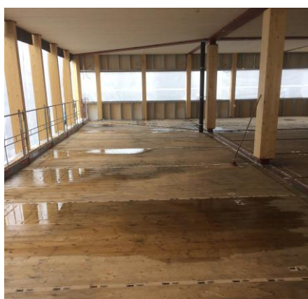
Fig. 5. On several occasions, water pooled on the floor structure. Precipitation ran down primarily from the above floor structures.
