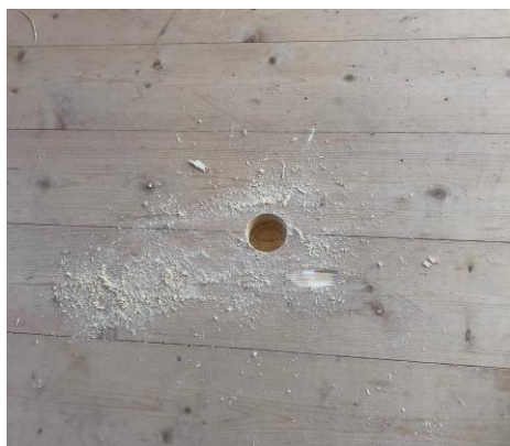
Fig. 9. Sample taken with a core drill in the connection gap between two timbers from the top of the floor structure (CLT).
