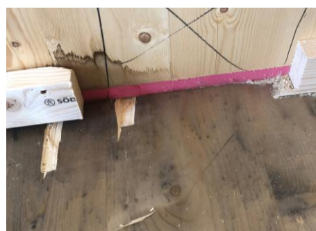
Fig. 8. Sample taken from the top side of the floor structure (CLT) under the sound and vibration pads and inner walls (CLT). The surfaces have been stained primarily by discoloured water.
