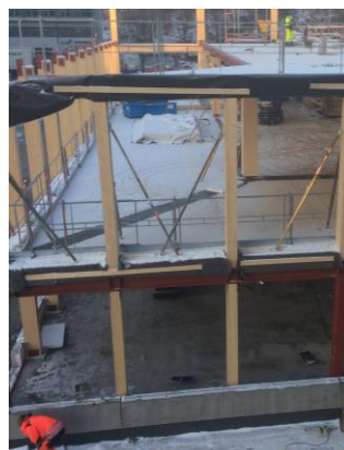
Fig. 2. Frame construction at the case study in west Sweden and snow on the floor structures. Assembly of CLT frame without weather protection.
