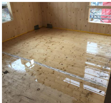
Fig. 6. Pooled water on floor structure in central Sweden. Precipitation ran down from the above floor structures.
