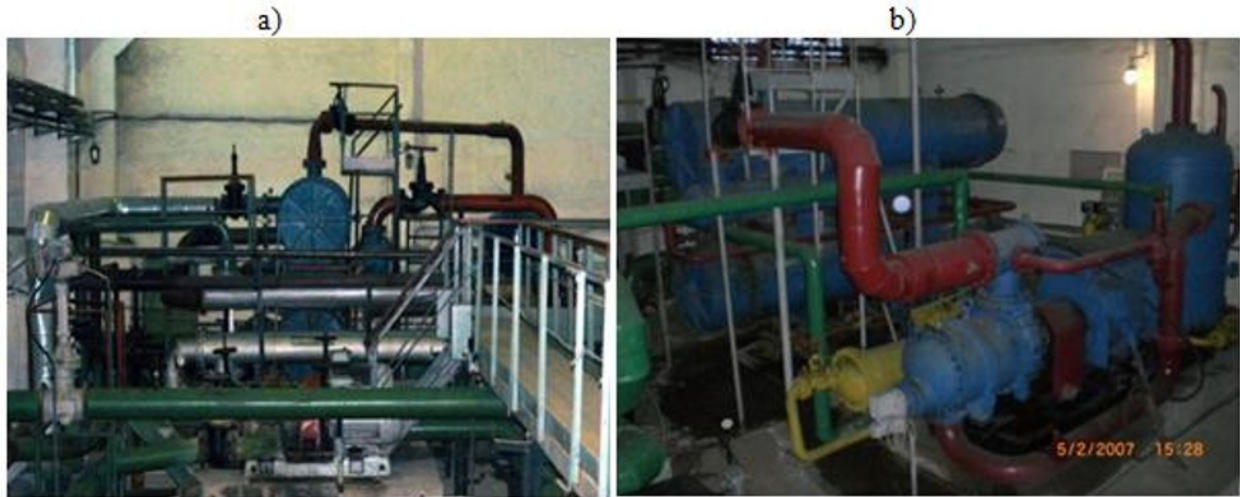
Fig. 5. The first industrial NT-3000 heat pump at Kazzinc JSC in the Republic of Kazakhstan.
