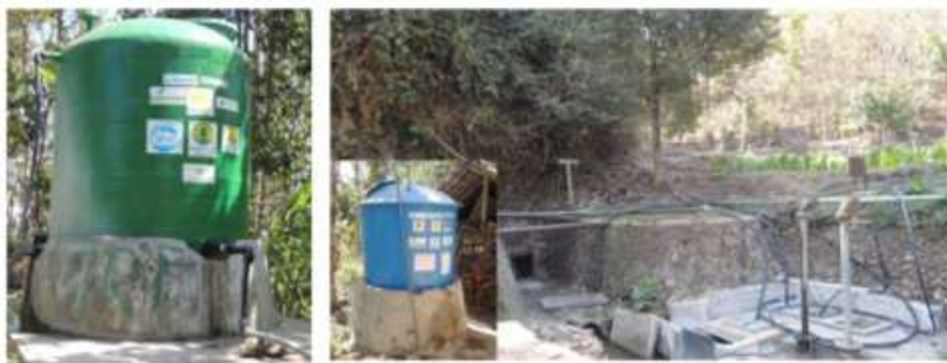
Fig.3. Solar water pumping system in Banyumeneng I hamlet, special region of Jogjakarta (source: kabarhandayani.com)
