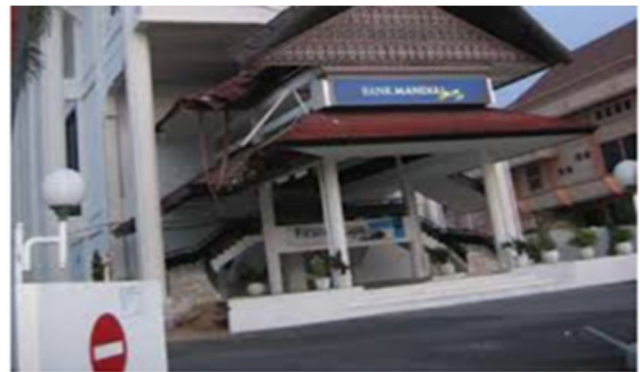
Fig. 1. Damage due to Liquefaction in Bengkulu City after the 2007 Earthquake [8]
