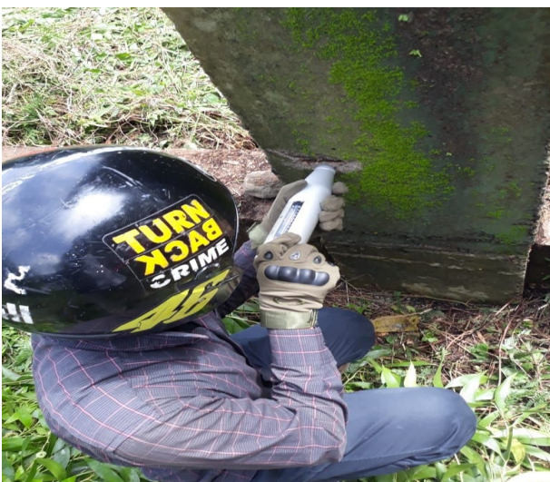
Fig. 3. The Concrete Surface is Overgrown with Moss
