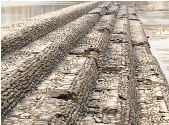
Fig1. Barrage damage map
