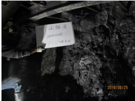
Fig. 1. Vault Surrounding Rock of Tunnel Face ZK41+088 of Left Line.
