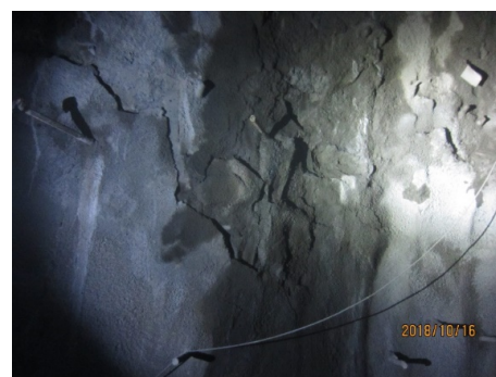
Fig. 4 Severe Arch Frame Deformation
