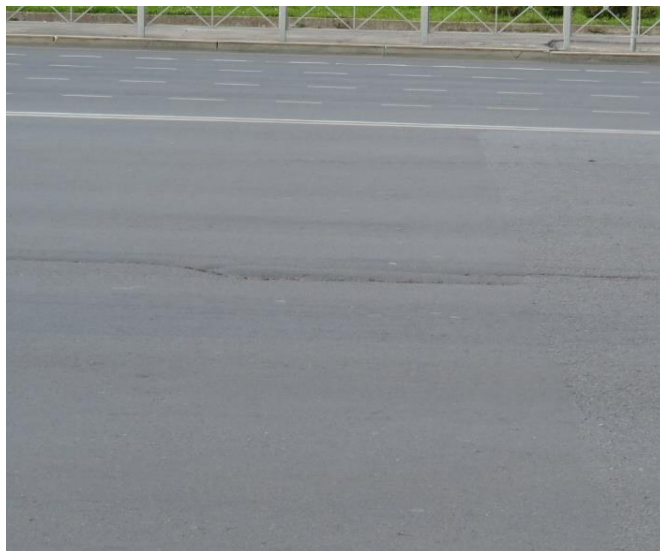
Fig. 2. Destruction of the roadway surface in the area of the EJ
