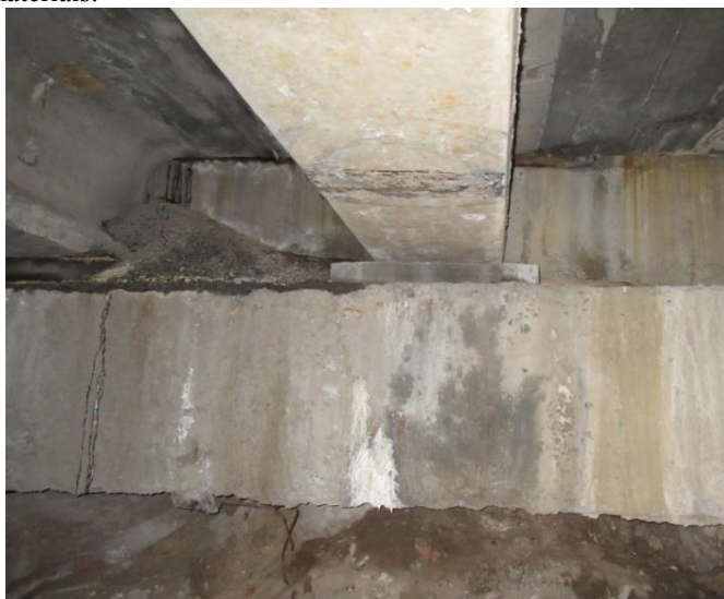
Fig. 1. Water ingress on the supporting parts of the bridge structure
