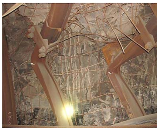
Fig. 6. Deformation of the frame stays.
