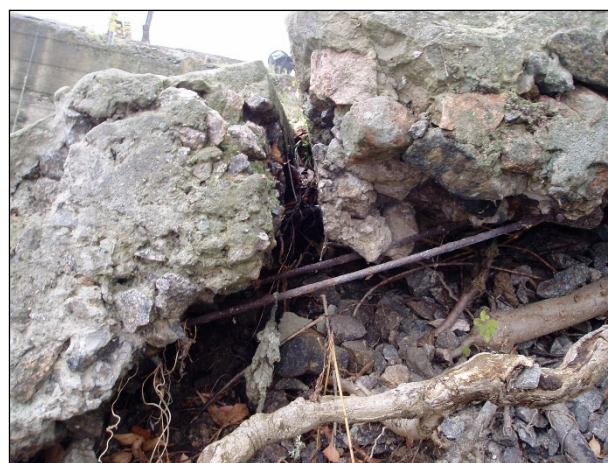
Fig. 3. Damaged area of the waterside protection.
