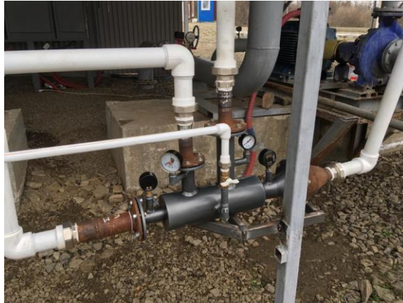
Fig. 5. Introduction of mineral fertilizers into the suction pipeline of the pumping station using a four-component jet mixer (photo by S. Tarasyants)
