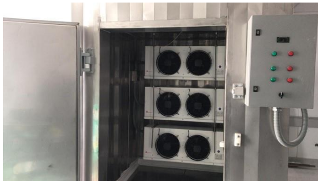
Fig. 2. Picture of the refrigeration chamber.
