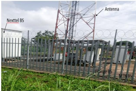
Figure 2: Telecom antenna located at the University of Buea, Southwest region Cameroon.
