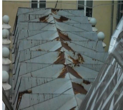
Fig. 5. View of through corrosion damage of steel roofing sheets.
