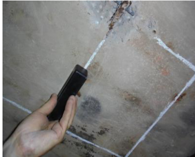
Fig. 7. View of the control of the reinforcing scheme of reinforced concrete elements by the magnetometric method.
