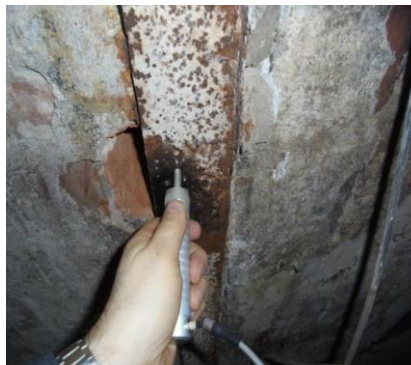
Fig. 8. Hardness testing of steel structural elements by ultrasonic contact impedance using the TKM459S device.
