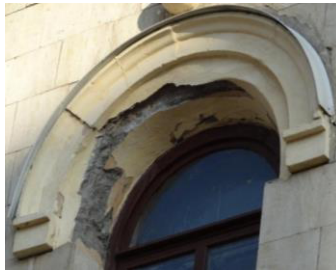
Fig. 2. View of defrosting and falling of decorative elements of window frames and masonry.
