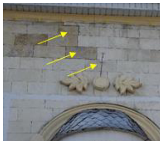
Fig. 3. View of inclined cracks in the facade wall.
