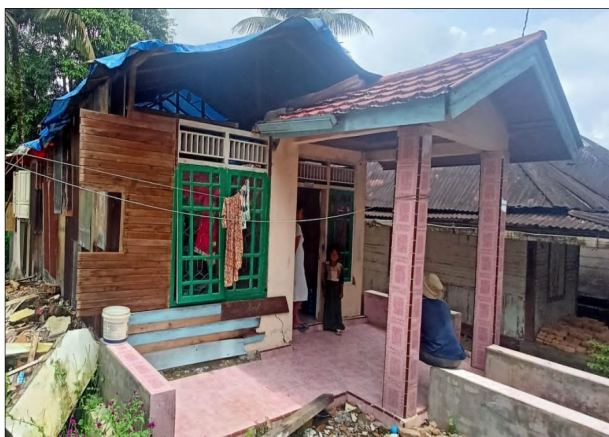
Fig. 4. Heavily damaged house.
