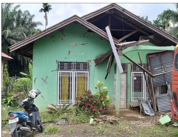
Fig. 3. Moderately damaged house.
