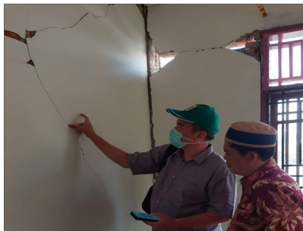
Fig. 5. Checking the damaged house.
