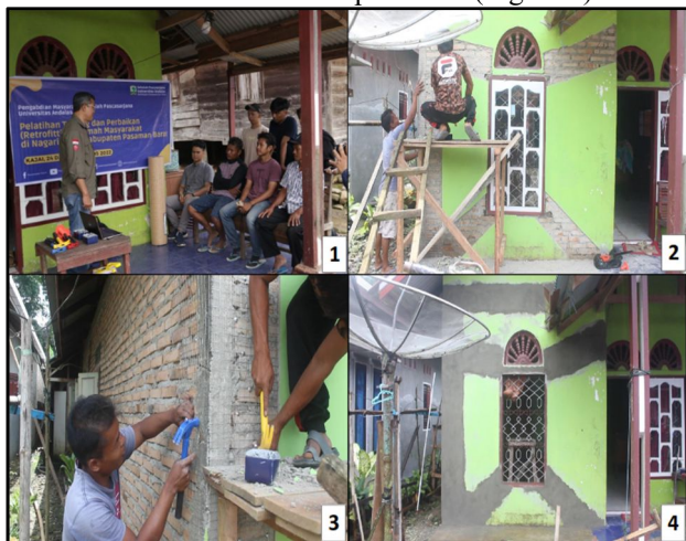
Fig. 7. Worker's training; Reciprocal stripping of stucco on cracks; The wall, the corner of the wall meeting has been peeled and ready to be installed with wire mesh; and the wall after the reciprocal wire mesh is installed and ready to be plastered.
