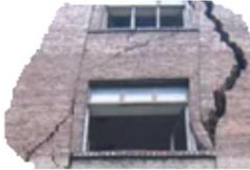
Fig.1. Linear and torsional character of destruction in the form of vertical, horizontal and inclined cracks from dynamic impacts.
